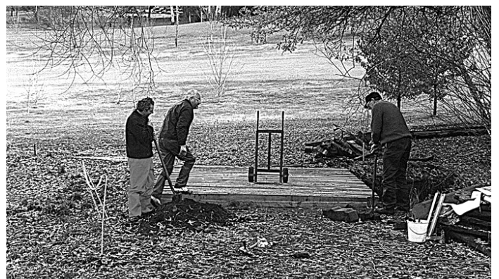
The new "Walker's Crossing" being constructed by Tom Hands, David Beck and Colin Mulrone in 1997.
